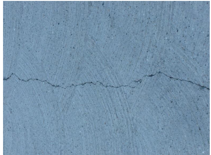
(b) Restraint crack, long and few in number (P751)
