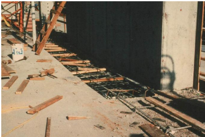
(a) Detail of delay strip at connection to wall. There is a gap between the end face of the wall and slab (P792)
