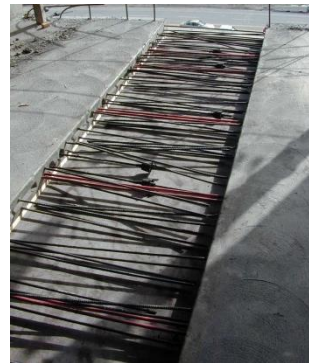
(b) Delay strip after concrete on both sides has been cast (P764)
