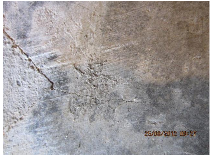
(b) Crack formation at construction joint (P759)
